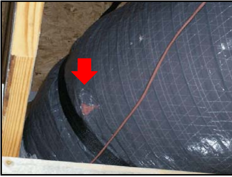
(20) Small tear in the supply duct above the air handler location.
