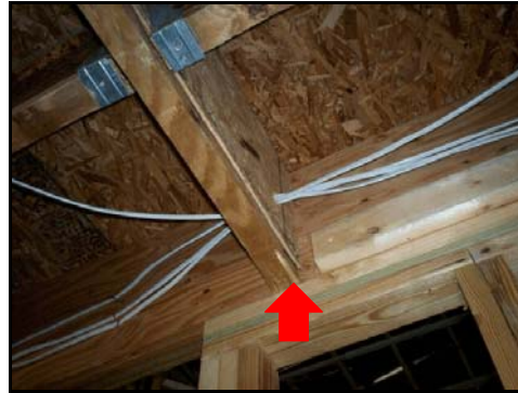
(15) NO bucket for short header beam between TJI's? Toe nailed?
