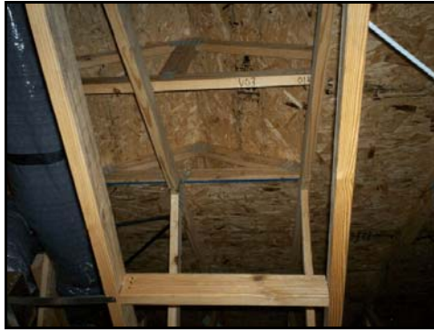
(21) No light at attic access
