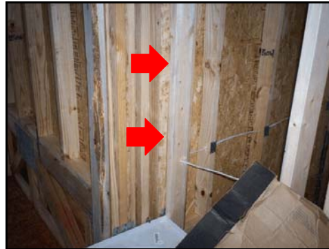
(18) Recommend nailing corner studs at bath / shower locations
