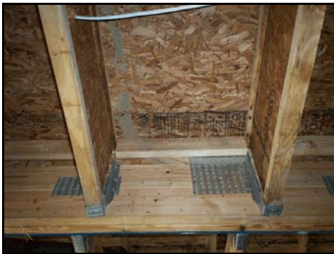
(8) Gaps between floors at the right wall / girder between bedroom #6 and right side of family room.
