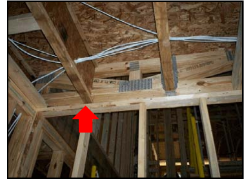
(16) No bucket for J21 TJI at right wall of garage door hall. Right TJI has bucket??
