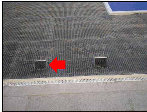
(9) Remove pest screen from dryer vent.
