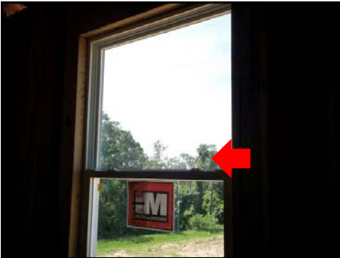
(17) Replace broken on right side of front right guest bedroom.
