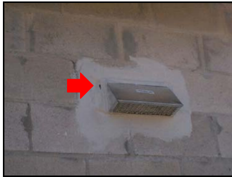
(5) Void in the sealant at the kitchen exhaust hood.
