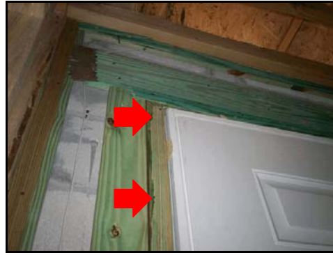
(12) Address the furring strips around the interior of the front door.
